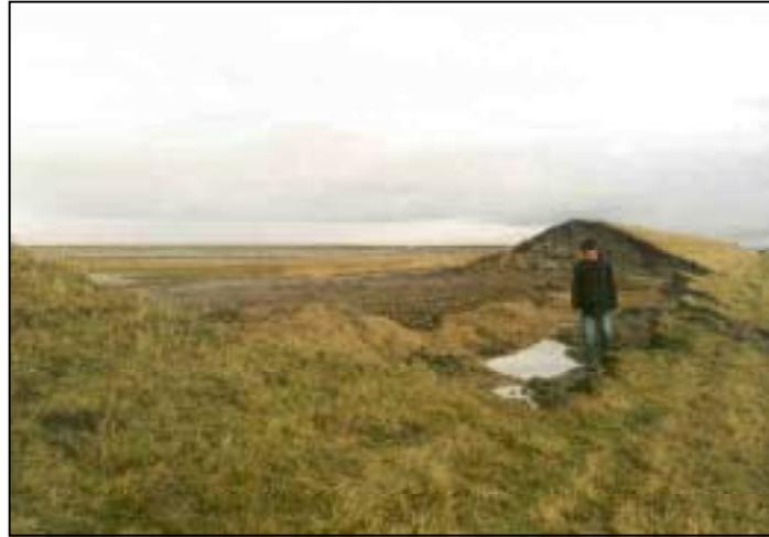
Fig. 1. Total Dike break on the island of Romo /Denmark(photo: Piontkowitz)
